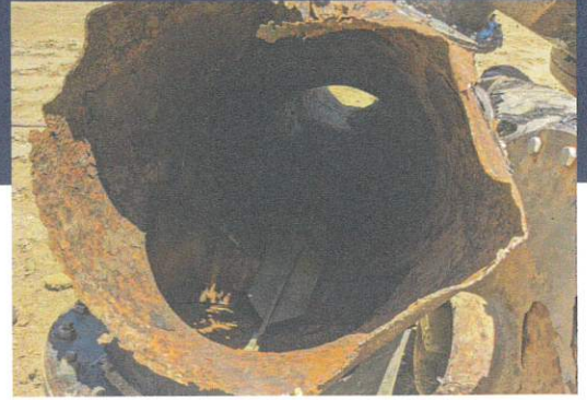
▲ 1962 severely corroded welded steel pipe recently removed from Sacramento river levee
