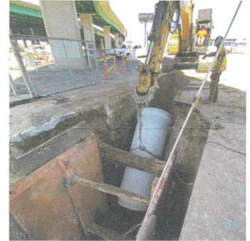
Installation of 42" reinforced concrete pipe to replace an old pipe beneath 3rd Street ▶
