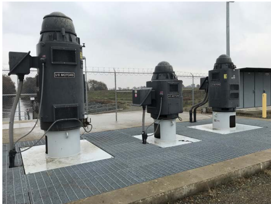
Figure 5 - Pumping Plant 2 Pumps
