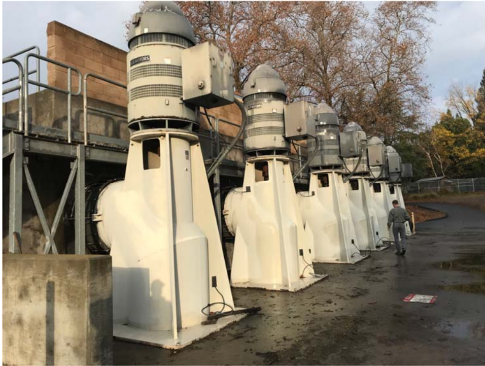
Figure 2 - Pumping Plant 1B Pumps
