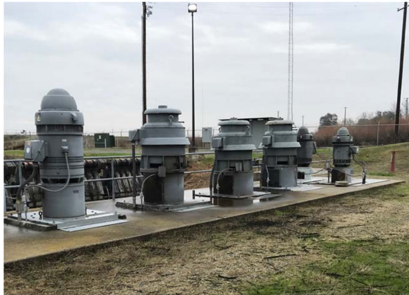
Figure 6 - Pumping Plant 3 Pumps
