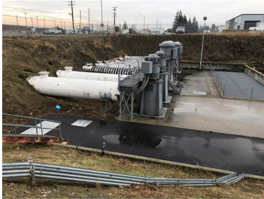
Figure 7 - Pumping Plant 8 Pumps
