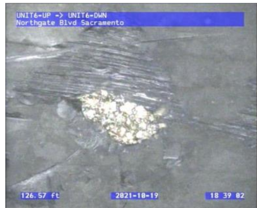
Photo 1-4. Suspected hole on unit #6 pipe.
