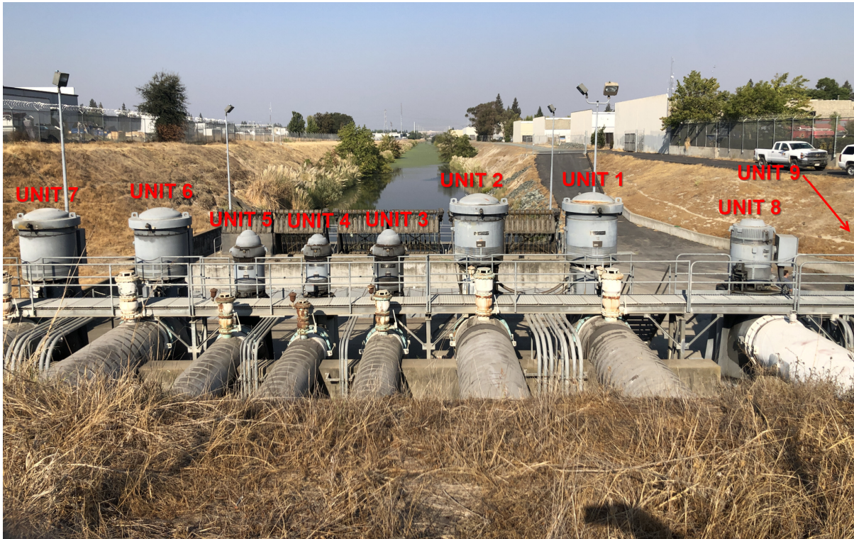
Figure 2-8 Original Discharge Pipes
