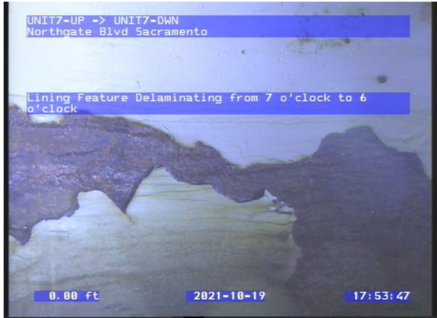
Figure 4-2 Epoxy Lining Delamination and Corrosion
