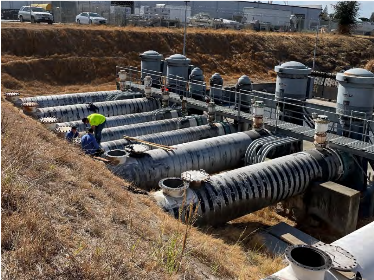
Figure 2 RD 1000 Pumping Plant 8 Showing the Blind Flange Entry Point
