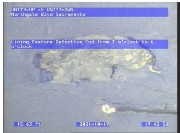
Photo 1-2. Spall on unit #3 pipe.
