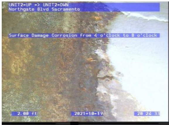
Photo 1-1. Heavy corrosion on unit #2 pipe.
