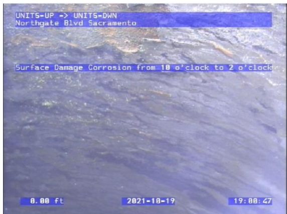
Photo 1-3. Corrosion on unit #5 pipe.
