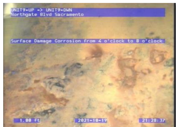
Photo 1-6. Corrosion on unit #9 pipe.
