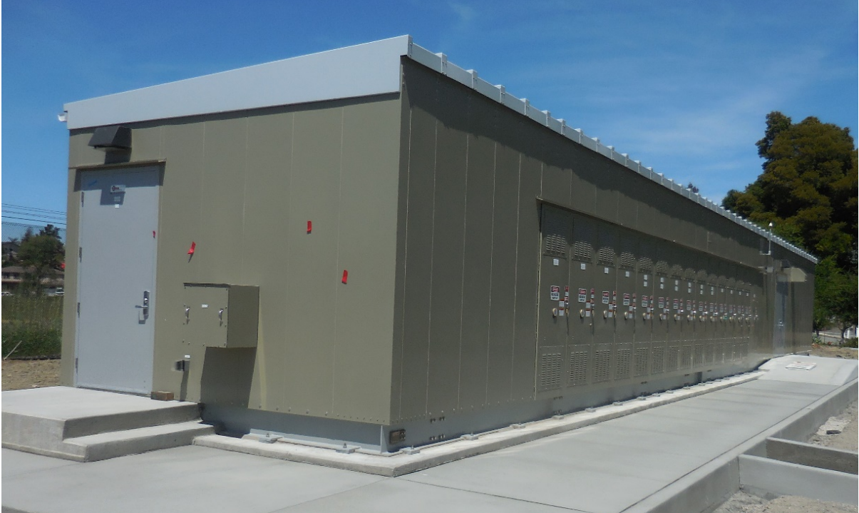
Figure 5-2 Integrated Power Assembly House
