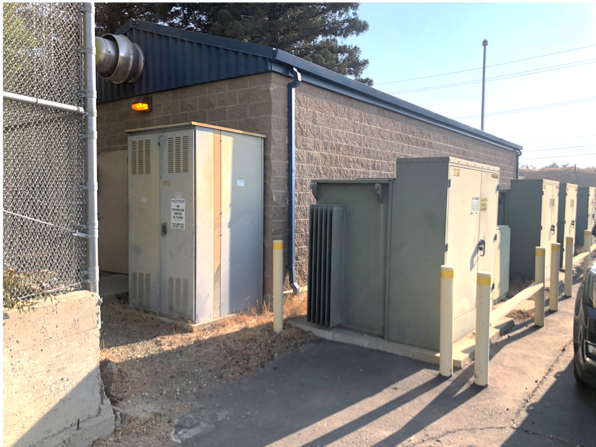
Figure 2-9 Instrumentation and Electrical Building
