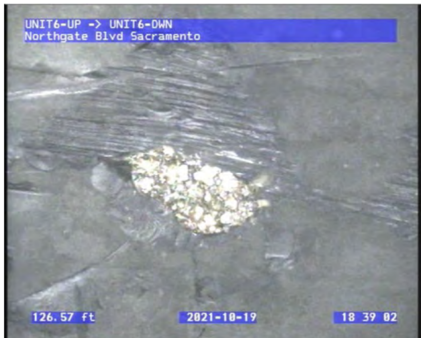
Figure 4-3 Pump 6 Pipe Wall Hole
