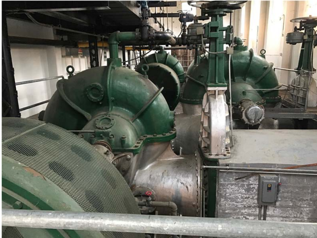
Figure 1 - Pumping Plant 1A Pumps
