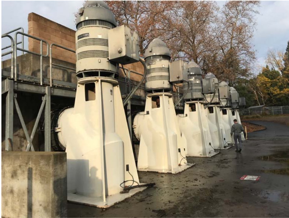
Figure 2 - Pumping Plant 1B Pumps
