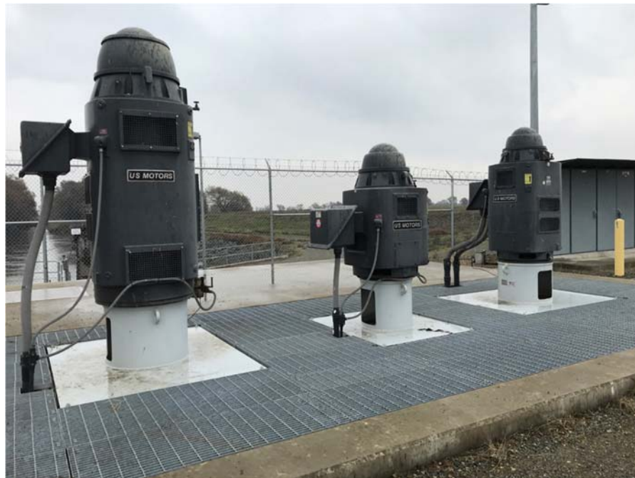
Figure 5 - Pumping Plant 2 Pumps
