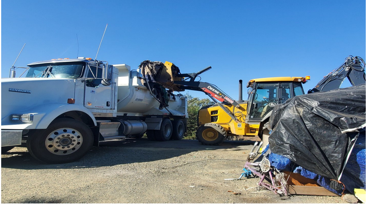
This particular location is just south El Camino, which shows our Distirct backhoe loading garbage and debris into the 10yd dump truck.
