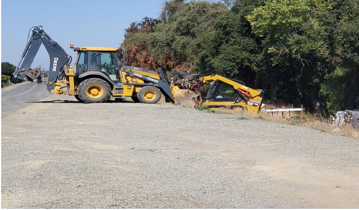
This picture shows a skid steer hauling trash from the levee toe, to the upper patrol road just south of San Juan Road.
